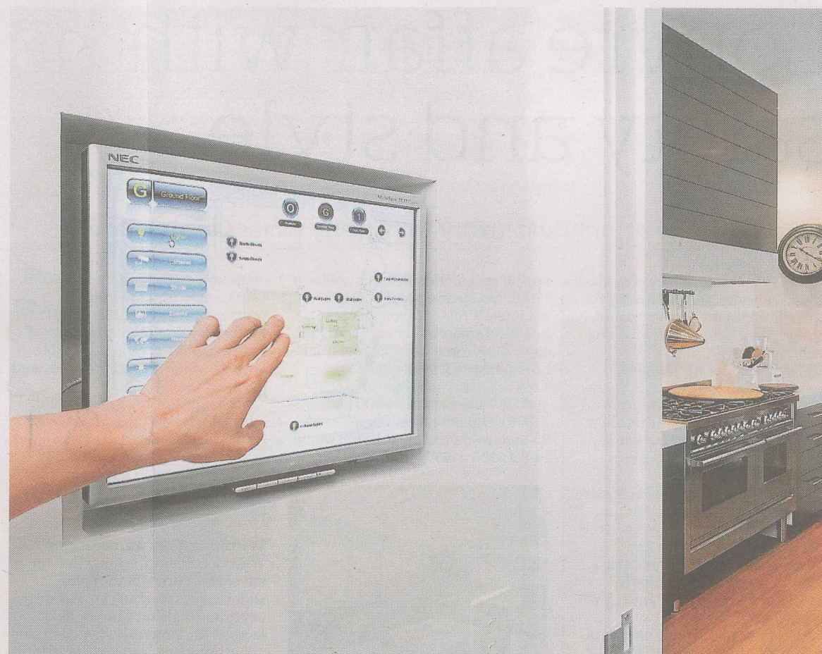
Peace of mind ... some security systems can send alerts to the home owner's smartphone. Photo: Michael Kai
